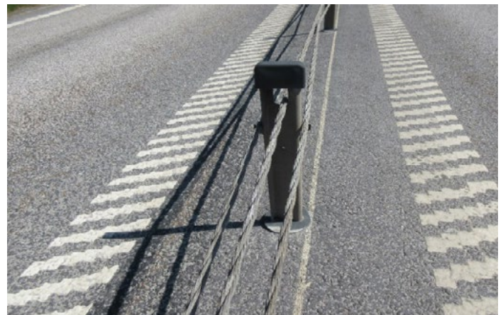
Wire rope lane dividing barrier (Photo -GEMS)
