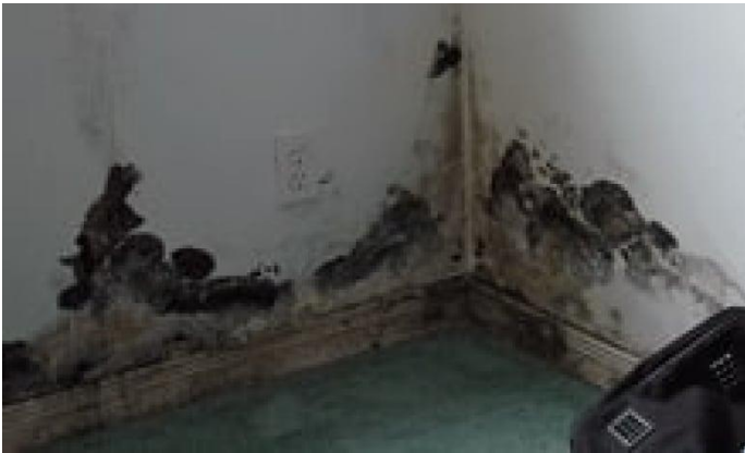
Mould in a home in Kashechewan FN after severe flooding in 2014. (CBC News, 2015)
